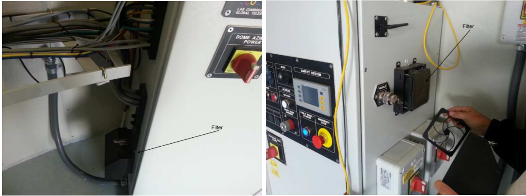
Filters on Control Cabinet
