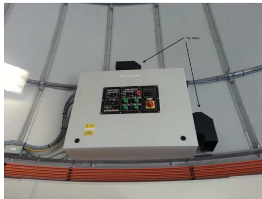
Roof control Filters
