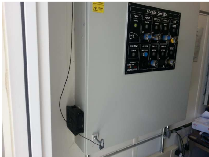
Filter on side of Access Control Panel
