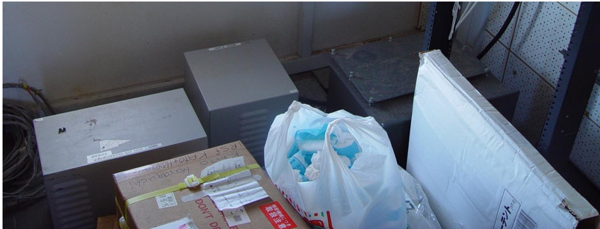
Figure 7: Three transformers in the Equipment room.
