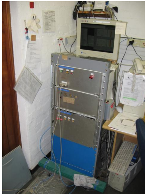
FIGURE 3: TELESCOPE CONTROL SYSTEM CABINET
