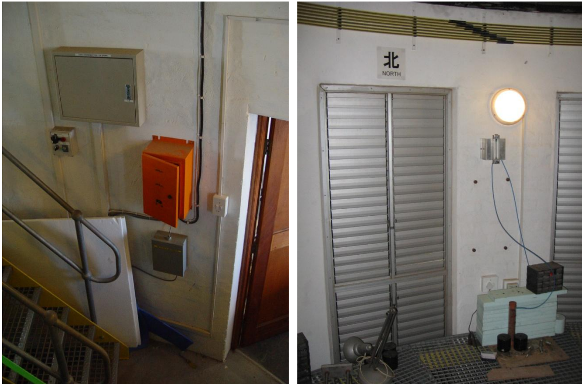
FIGURE 12: 100V AC DB (LEFT), FAN CONTROL
