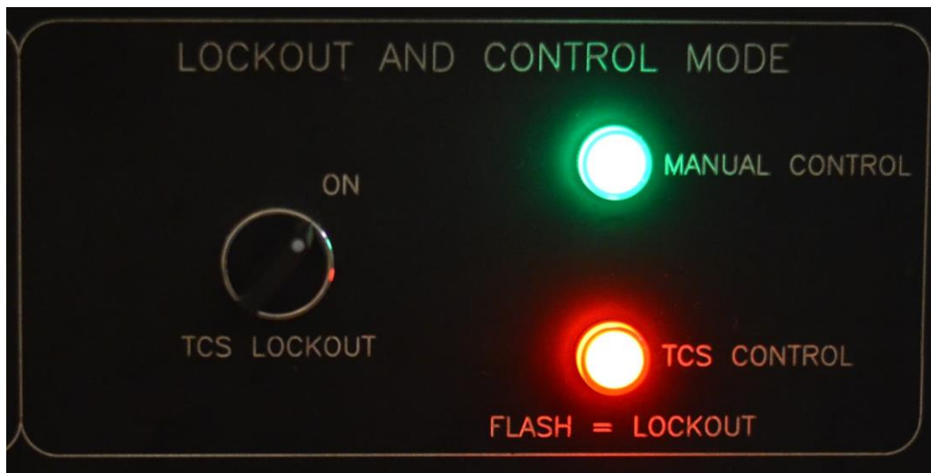
Figure 4: TCS LOCKOUT SWITCH
