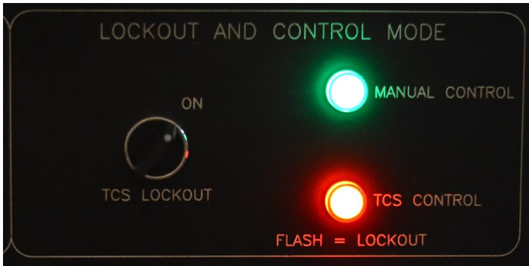
Figure 2: TCS LOCKOUT SWITCH
