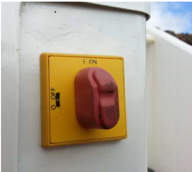
York Main Switch
