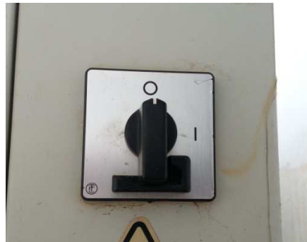
Chiller Main Switch
